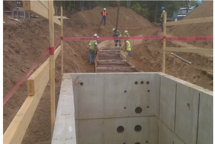
Crews work on an underground duct bank extending from a typical 8'x8'x24' vault
