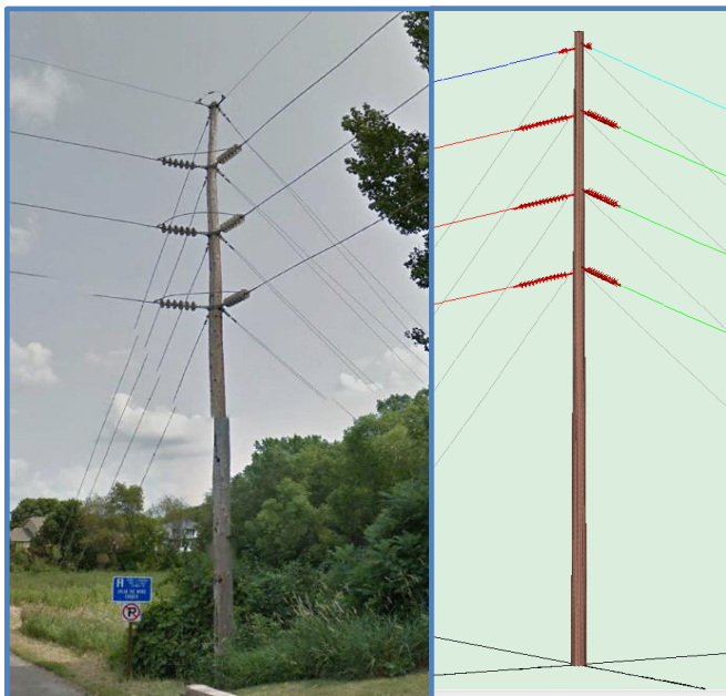
Typical Dead-End / Angle Structure
