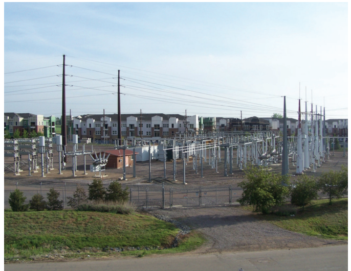
Typical Substation Layout: Broomfield Substation located near the intersection of Wadsworth Boulevard and 116th Avenue (approximately 6.8 acres).
