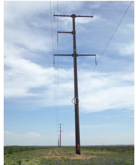
Example of 69-kilovolt structure. Structure types can differ based on route selected and other factors.
