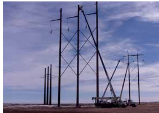
After setting structures, crews work on stringing conductor on the new transmission lines.
